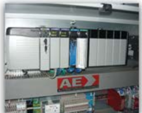
Reliable PLC Controlled Networks
